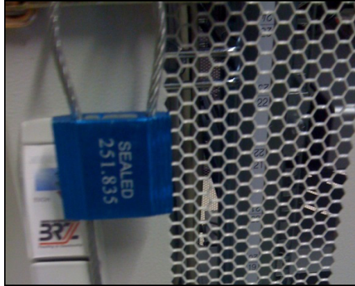
Figure 4: Sealed security rack
